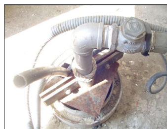
Check the water level measuring pipe
